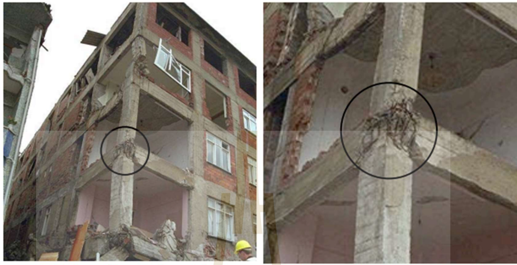
(a) Failure of beam-column joint (b) Close-up of beam-column joint failure (Image source: http://nisee.berkeley.edu/elibrary/Image/IZT-673 )
