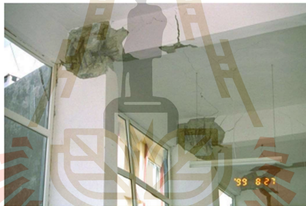
(c) Damage to beam-column joint of building under construction in Adapazari, Turkey (Image source: http://nisee.berkeley.edu/elibrary/Image/IZT-749 )
